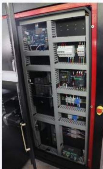
4 Circuit Control System
