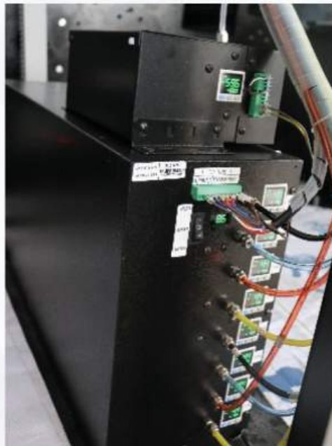
5 Negative Pressure System
