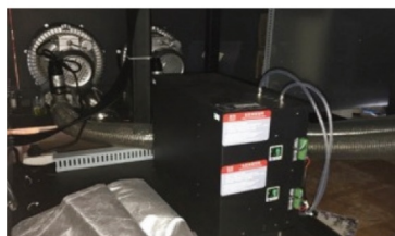
Negative Pressure System
